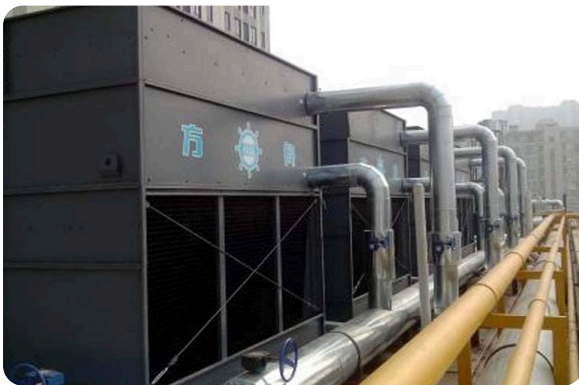
Industrial Furnace Recirculating Water Cooling Tower System image 2
